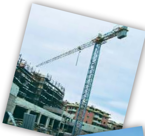
JIB TOP TOWER CRANE
